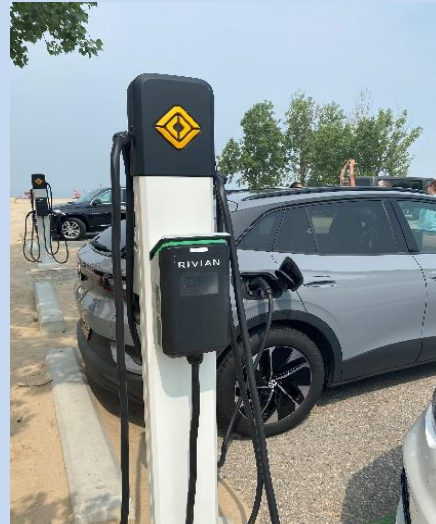
Car Charging Stations
