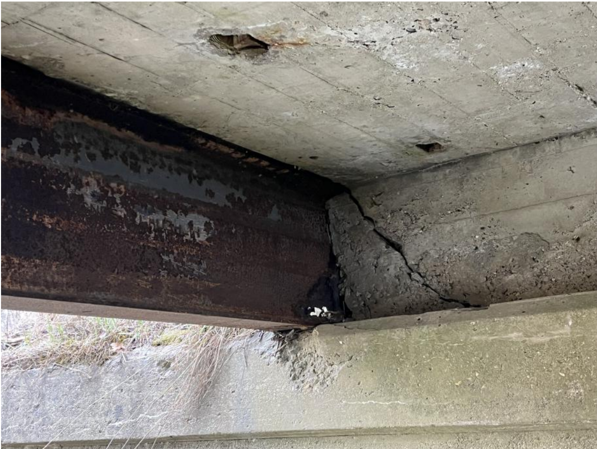
Hole in web of beam at south abutment. An additional three beams have holes in webs.
