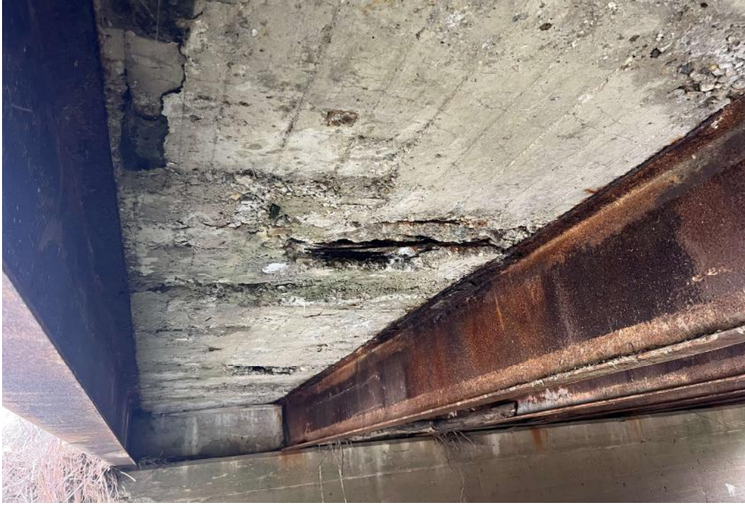
Spalling and delamination throughout deck underside
