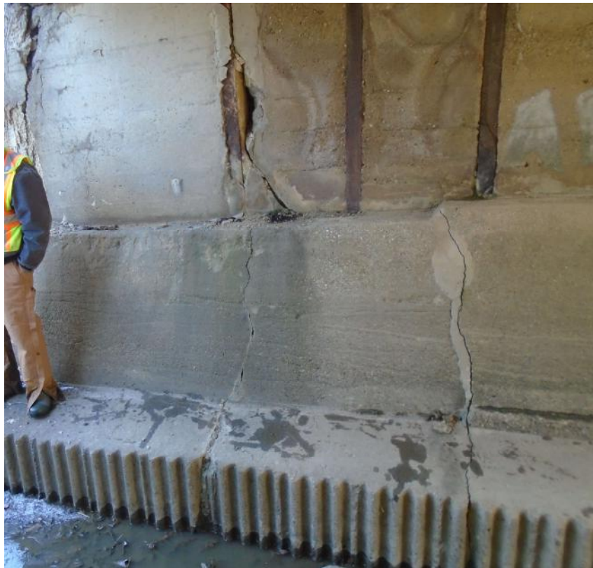
Abutment – Previous Repairs Cracked and Failing
