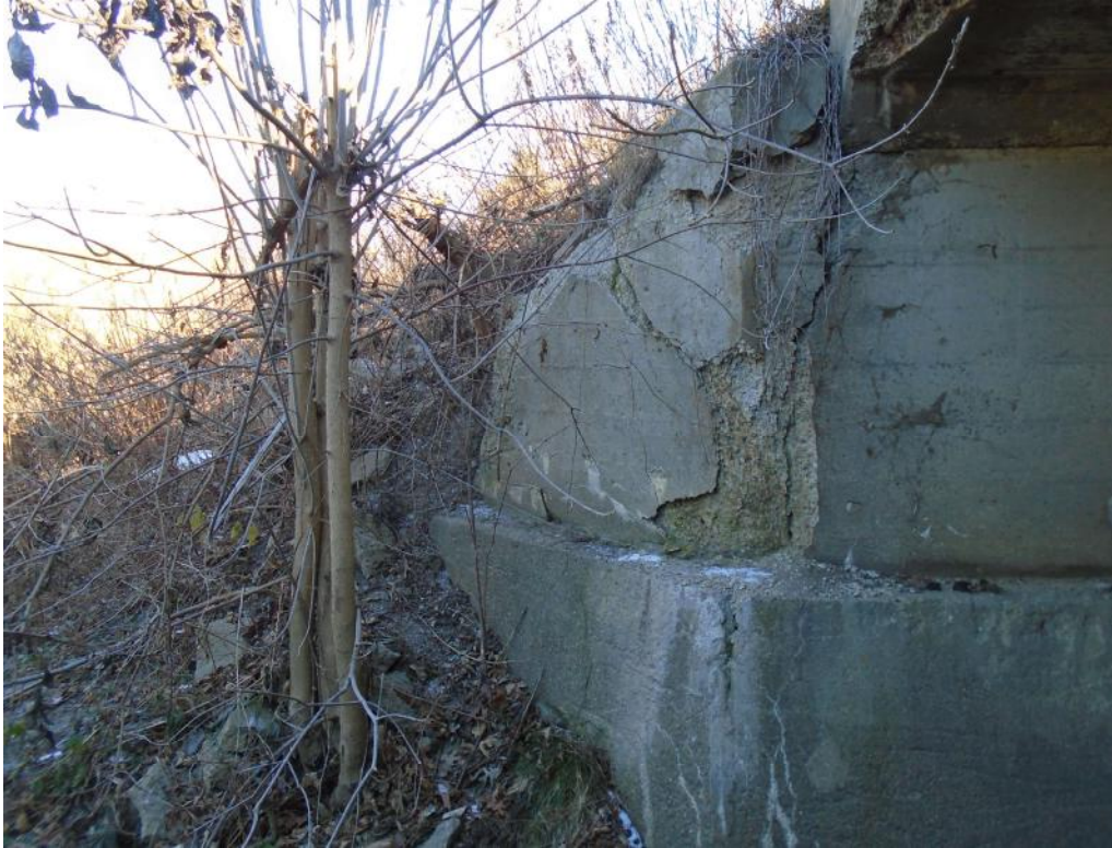
Abutment and Wingwalls – Concrete Crumbling
